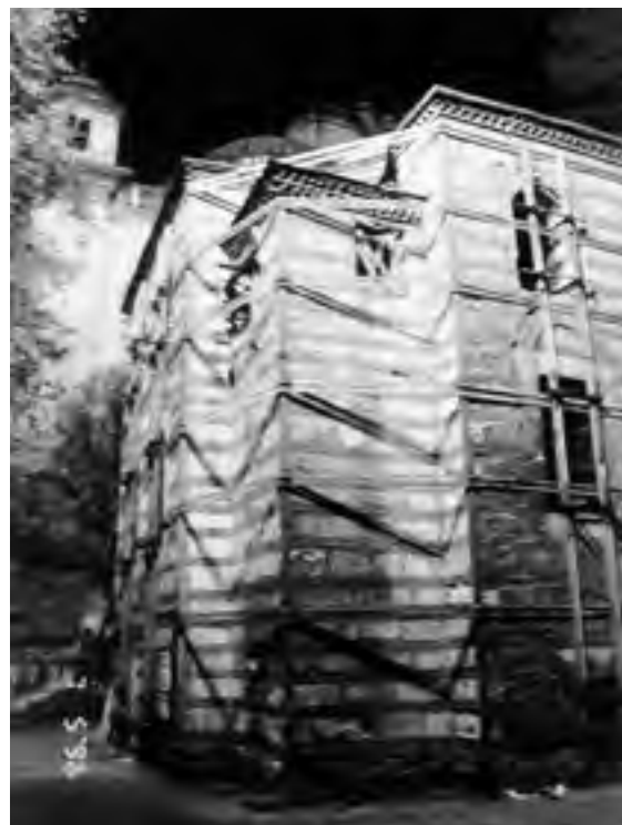
Fig. 12.57. Close-up view of the Church of Mehmed II the Conqueror. The building is gradually falling apart. To protect it, it was pulled together from all sides with iron reinforcement. Photo of 1996.
